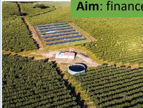
140 kWp – PV/Diesel - Drip Agro-industry Portugal
