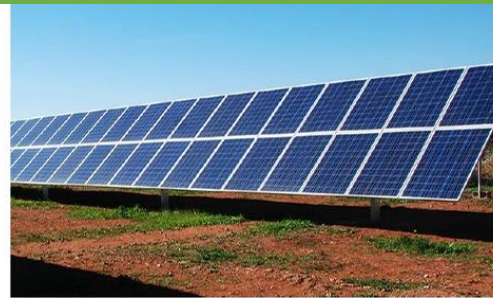
120 kWp – PV/Grid - Drip Agro-industry Morocco
